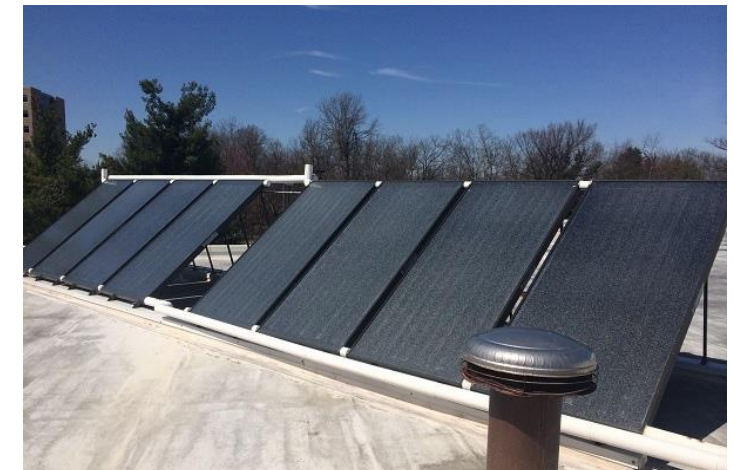
Bruce Poundstone Regulatory Services Solar Thermal Array
