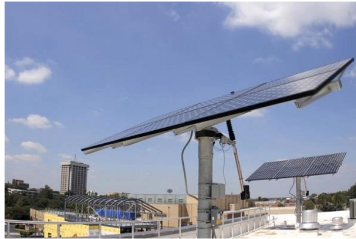
Davis Marksbury Solar PV Array
